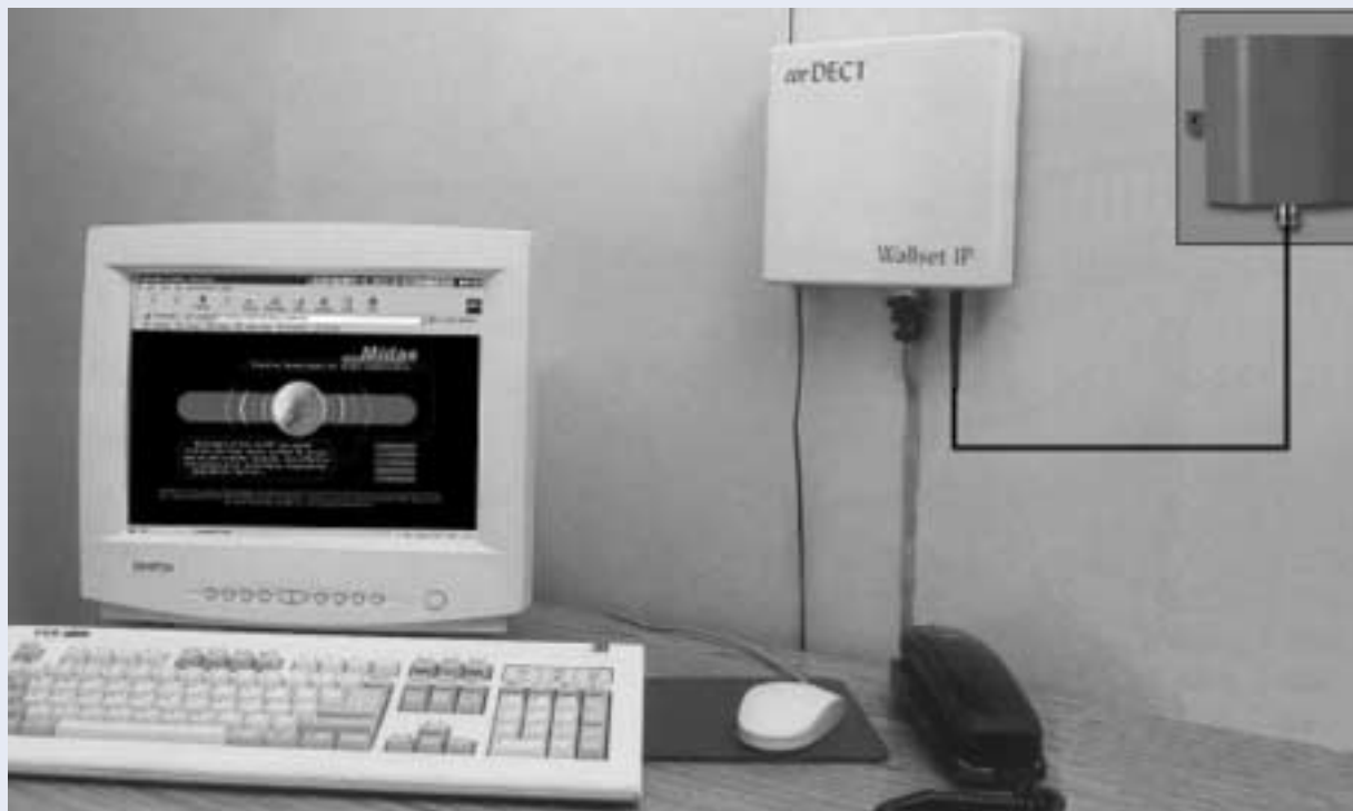
The corDECT wallset with PC and telephone connections and cabled to external antenna.
