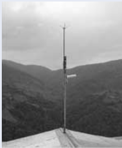
A customer-premises antenna and call-processing unit.
